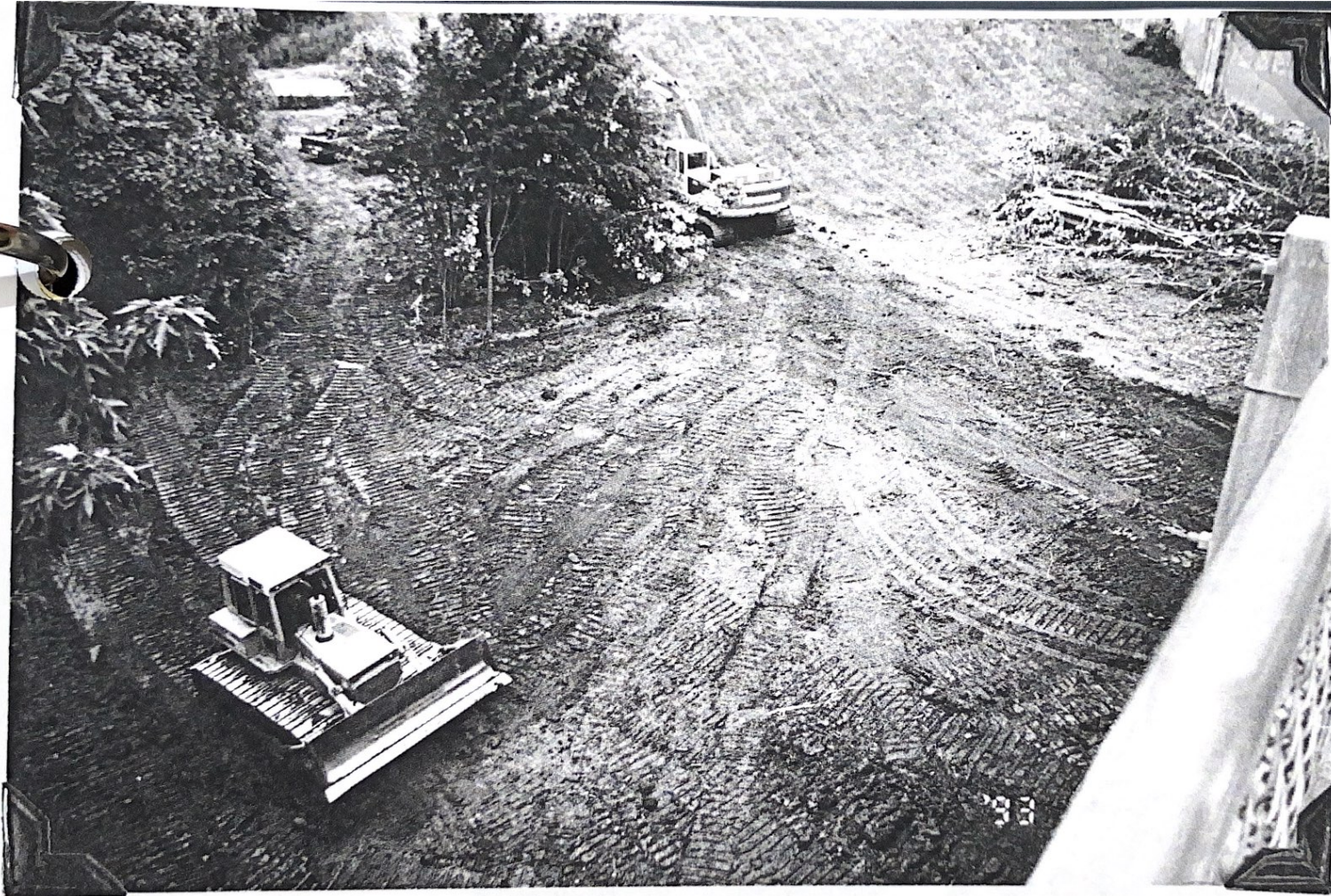
Earth movers clear the land, near the Newport - Covington Fifth Street Bridge, for the future home, of the Cincinnati Rowing Club.
